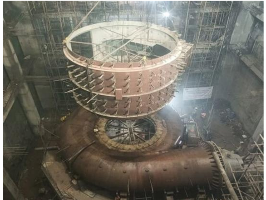
Machine Hall Unit 1 Spiral Casing
