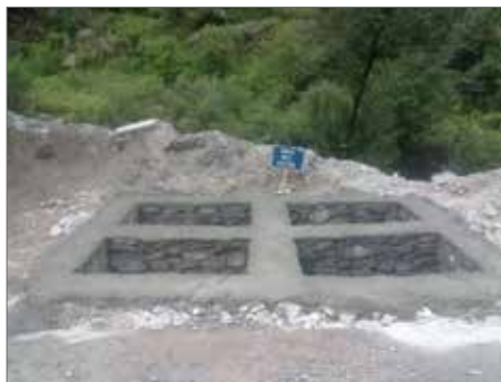
Food waste treated at decomposting pit
