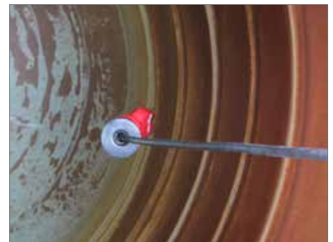
Flow Meter Installed in overhead water tank
