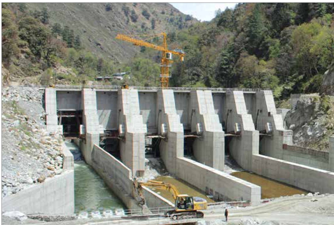
The barrage nearing completion at the 100MW Sainj Hydroelectric Power Project in Kullu district of Himachal Pradesh
