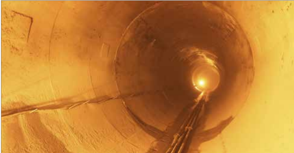
The 3.85m diameter Head Race Tunnel constructed using long distance concrete pumping methodology.
