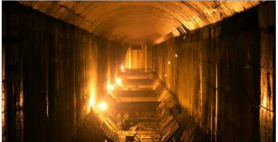
The desilting chamber of the underground water conductor system of Sainj Hydroelectric Power Project
