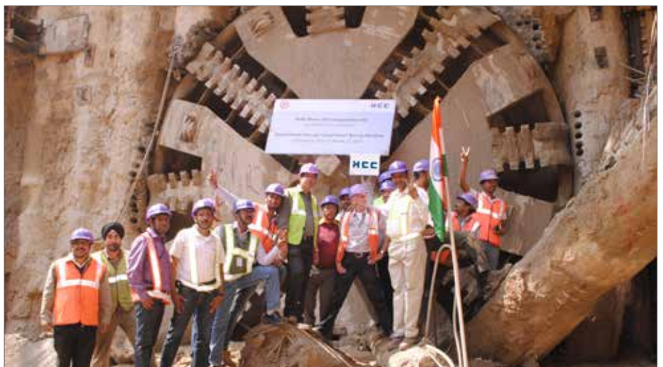
HCC team celebrating the break-through of up-line tunnel achieved on March 13, 2014 at DMRC's CC 30 project
