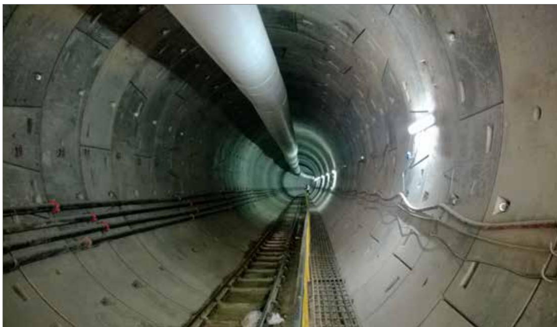
The 2.2 km twin-tunnel of DMRC's CC30 package, part of the 59km long Majlis Park to Shiv Vihar Metro Corridor of Phase III.
