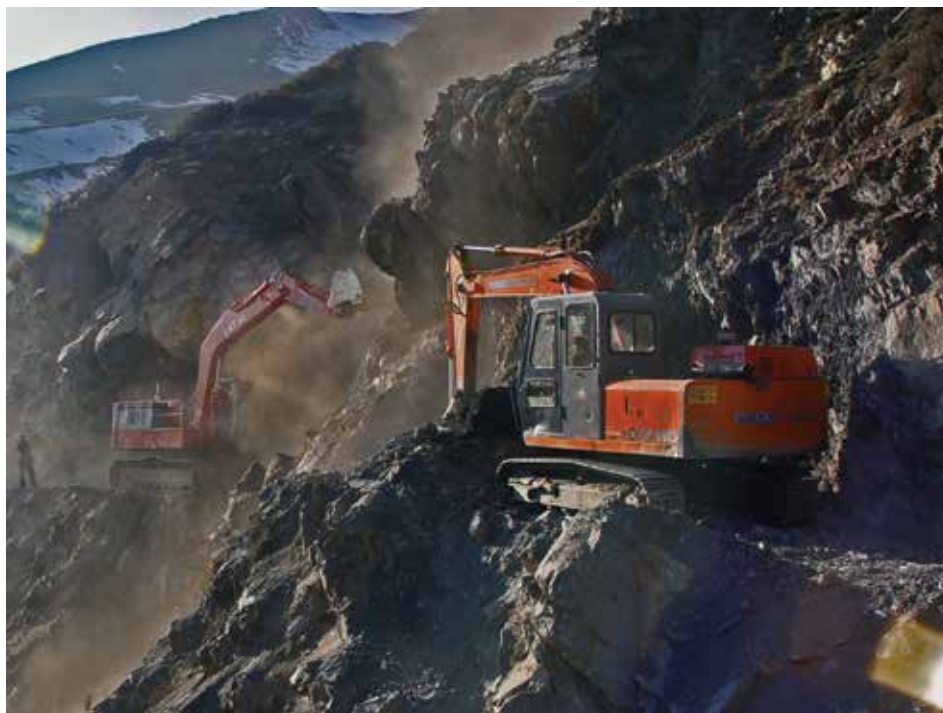
At Lalgulam, the team crossed a huge vertical cliff by moving excavators from the top of the hill .
